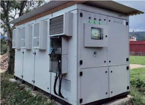
GRES Thermal Power Plant Project Country: Austria
